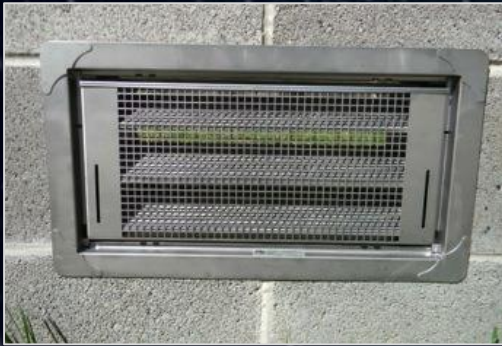
Flood door closed, obstructing the opening.
