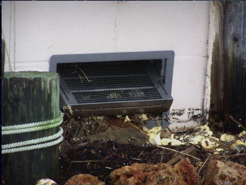
Pictured: Engineered flood vent following Hurricane Ida (2009)
